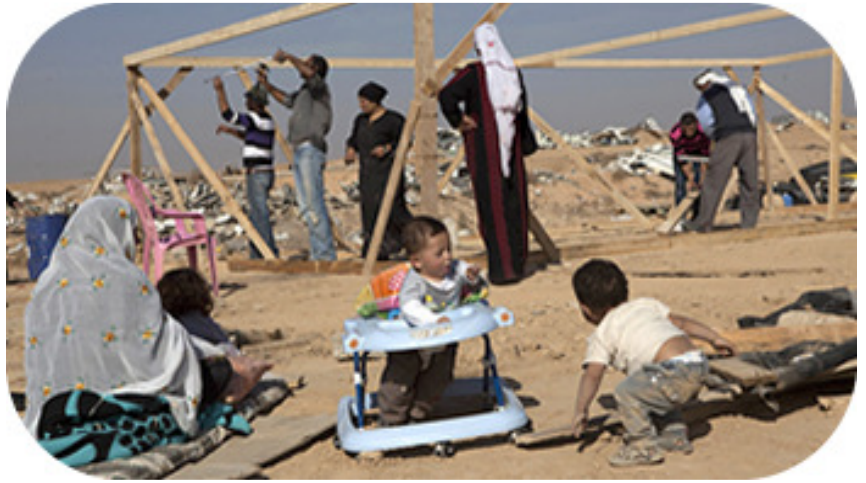
Rebuilding: Members of the Al-Turi family from the village of Al-Arakib rebuild a makeshift home in December after it was demolished for the eighth time by the Israeli government.
